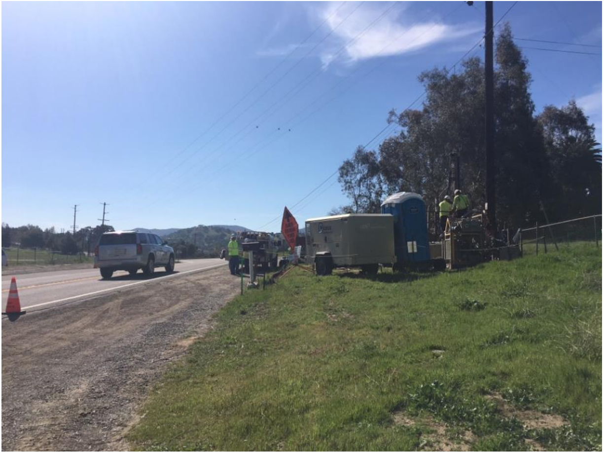
Photo 6: Crews were observed drilling micropile foundations at Pole Z118034 (TL682). Work activities remained within the work limits per MM BIO-1A. Traffic control crews were observed near the work limits with traffic cones and signs to direct traffic if required, per APM TRANS-02.
