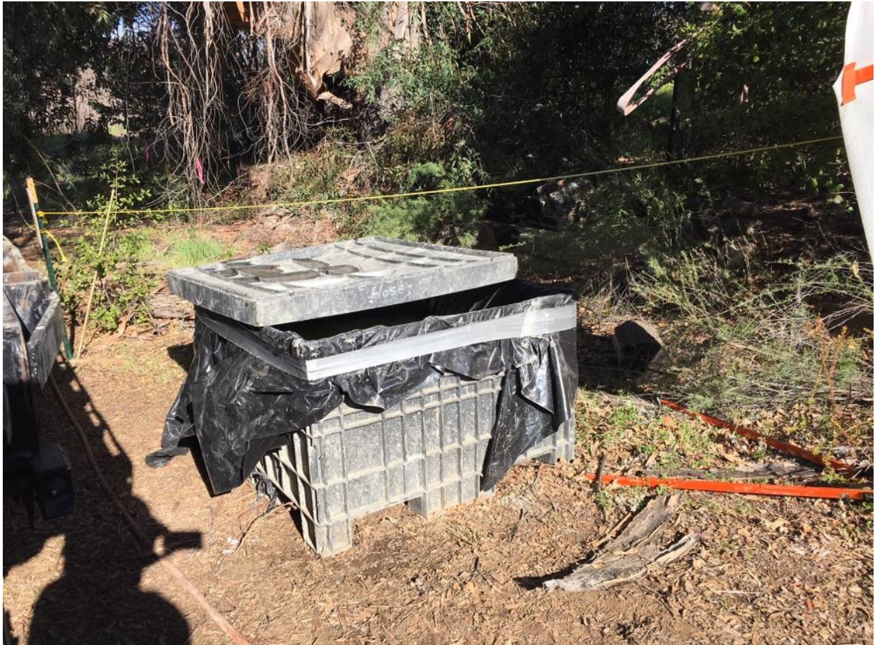
Photo 5: A lined concrete washout basin with cover observed near grouting operations at Pole Z118037 (TL 682), in accordance with APM HYD-01.
