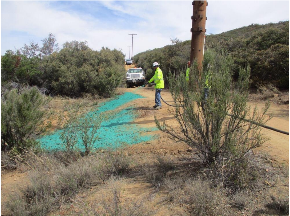
Photo 4: A crew is observed applying hydro-mulch at P176976 (C442) in accordance with the Erosion Control Plan and SWPPP.
