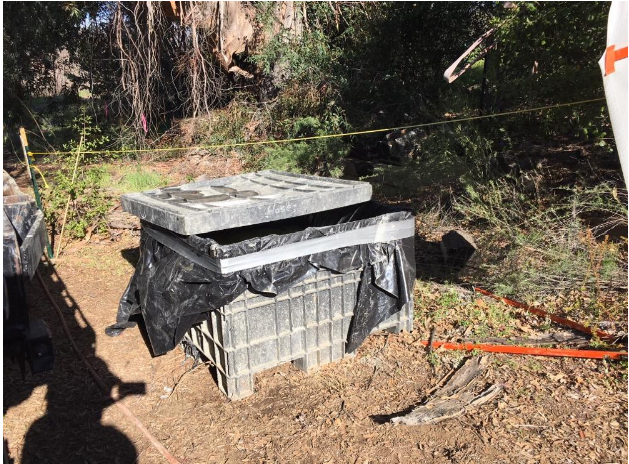
Photo 5: A lined concrete washout basin with cover observed near grouting operations at Pole Z118037 (TL 682), in accordance with APM HYD-01.
